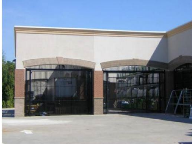
Figure 1113-B: The above image illustrates a facade wall and fence that is an extension of the principal building that is designed to screen outdoor storage areas.
