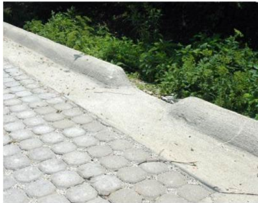
Figure 1115-A: Cuts in the continuous curb allow for stormwater to be directed into landscaped areas.
